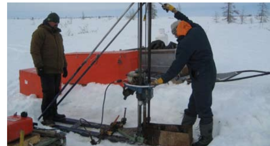
Drilling borehole for thermistor cable installation, peatlands near Fletcher Lake – Photo: Wendy Sladen
